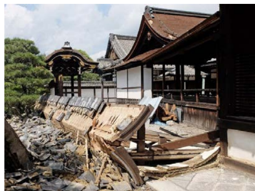
Damage to the Hongwanji's South Noh stage's outer wall. Jiji Press
