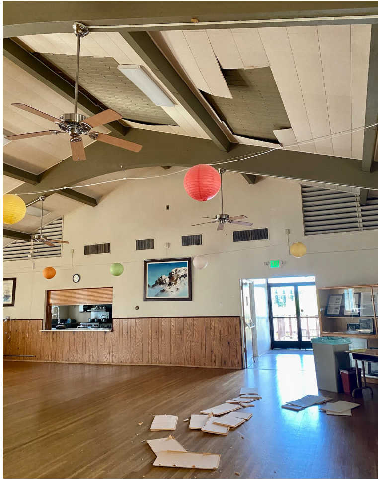
Fallen ceiling tiles in the Buddhist Temple of San Diego's social hall are shown after heavy rains pelted the Southern California region on Jan. 22. (Courtesy of Nancy Martinez)
